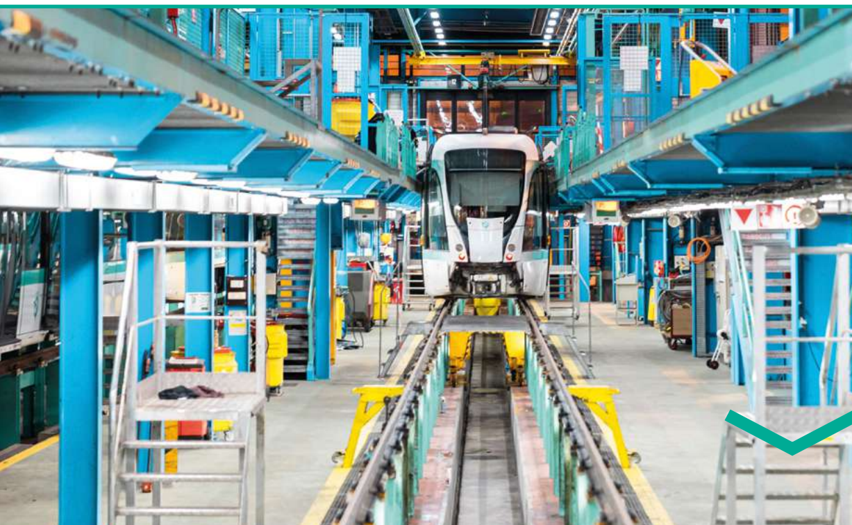
Tram line T2 maintenance and depot site at Issy-les-Moulineaux © RATP - Hamdi Chref
