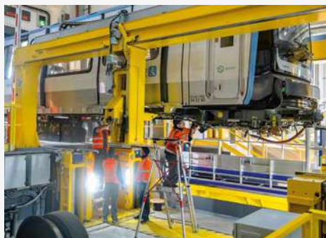
Metro line 11 train maintenance centre at Rosny-sous-Bois.
